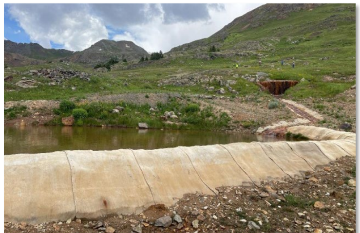
A berm constructed to manage surface water near the Sunbank Group Mine
