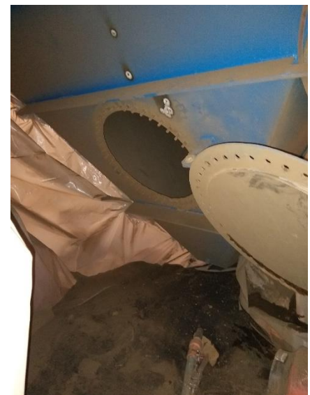
Clarifier prepped for work and in the process of having the lining removed from the inside.
