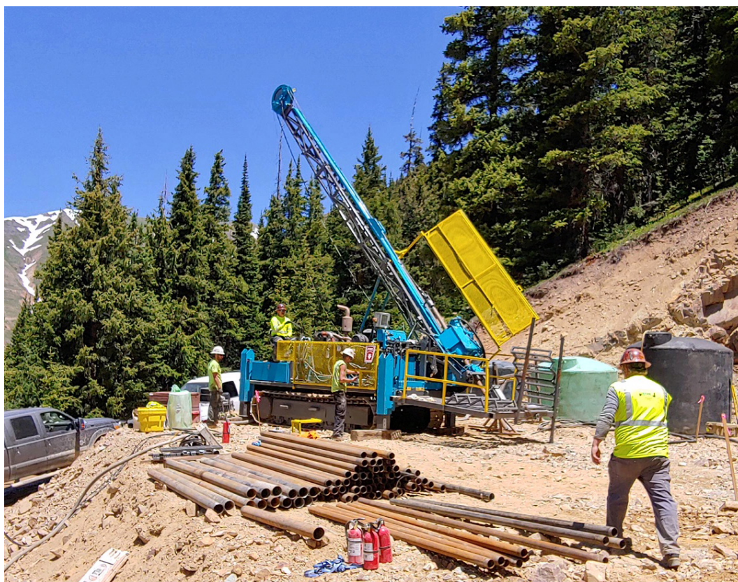
Setting up the drill rig to install a monitoring well into the American Tunnel.
